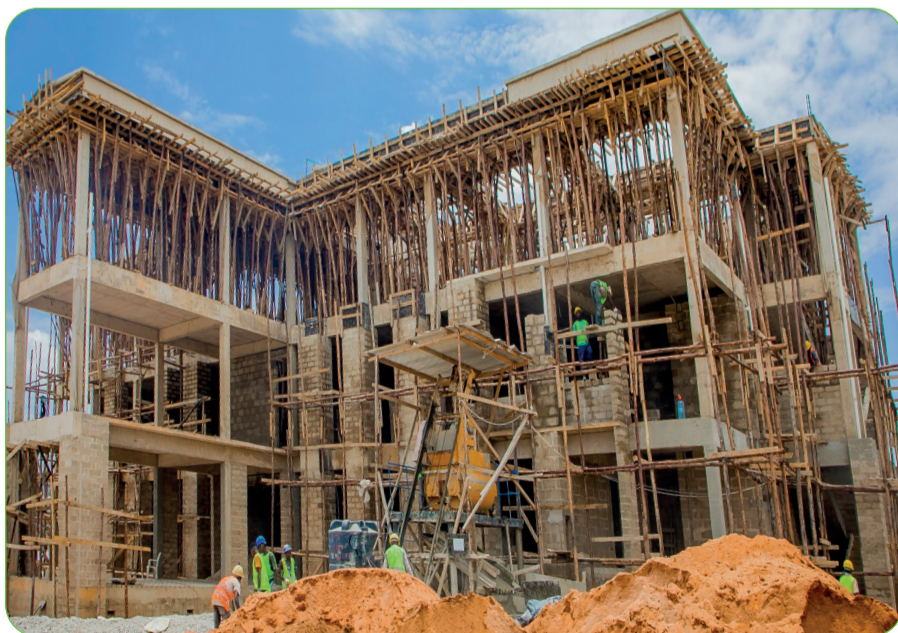
Construction of PPRA headquarters is progressing well in Dodoma as captured in the photo of March 10, 2023
